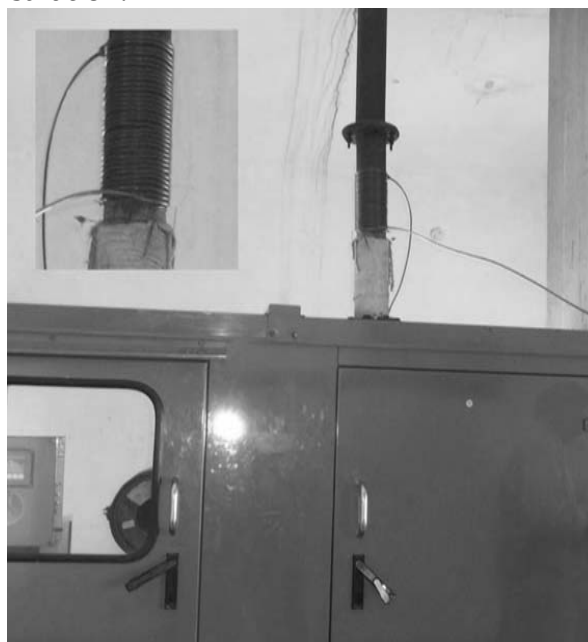
Fig.2 Waste Heat recovery from 140kVA DG set without thermal insulation
