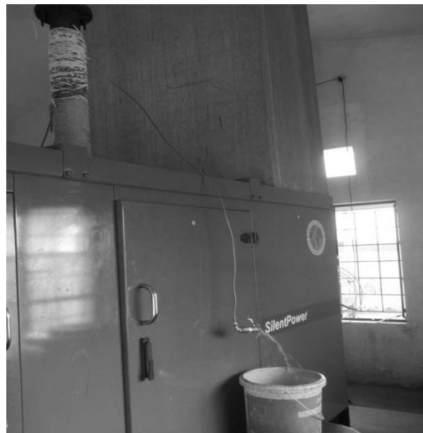
Fig.3 Waste Heat recovery from 140kVA DG set with thermal insulation
