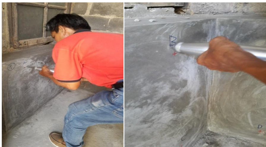
Fig 10. Shooting the points of simple masonry wall placed at the outer side of house wall (I-II series)
